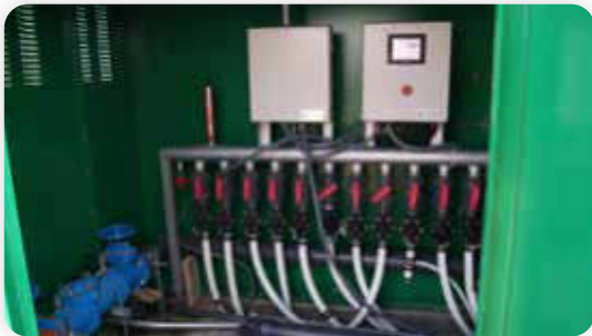
Drain away System
